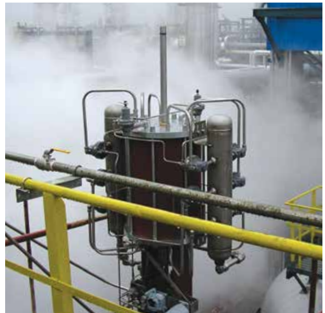
SVI II AP on steam conditioning valve
